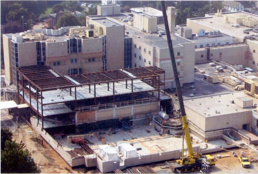
Beebe Medical Center, Lewes, Del., is finishing up a $35 million expansion. Construction will be complete this fall. Photo courtesy of Beebe Medical Center.
