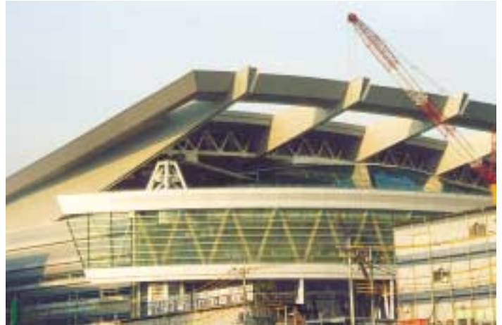
When the 20-minute conversion begins, an automatic, flexible utility regulation system starts up as the 64 base bogeys, or trucks, travel their steel rails. Electric cables wind up and release from their reels. Plumbing and air-conditioning supplies cut and reconnect.
